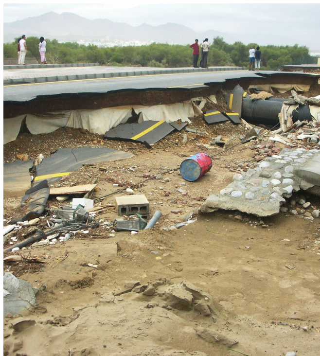
Damages in Muscat after the passage of Cyclone Gonu, Oman, 2007. Source: Wikimedia Commons.
